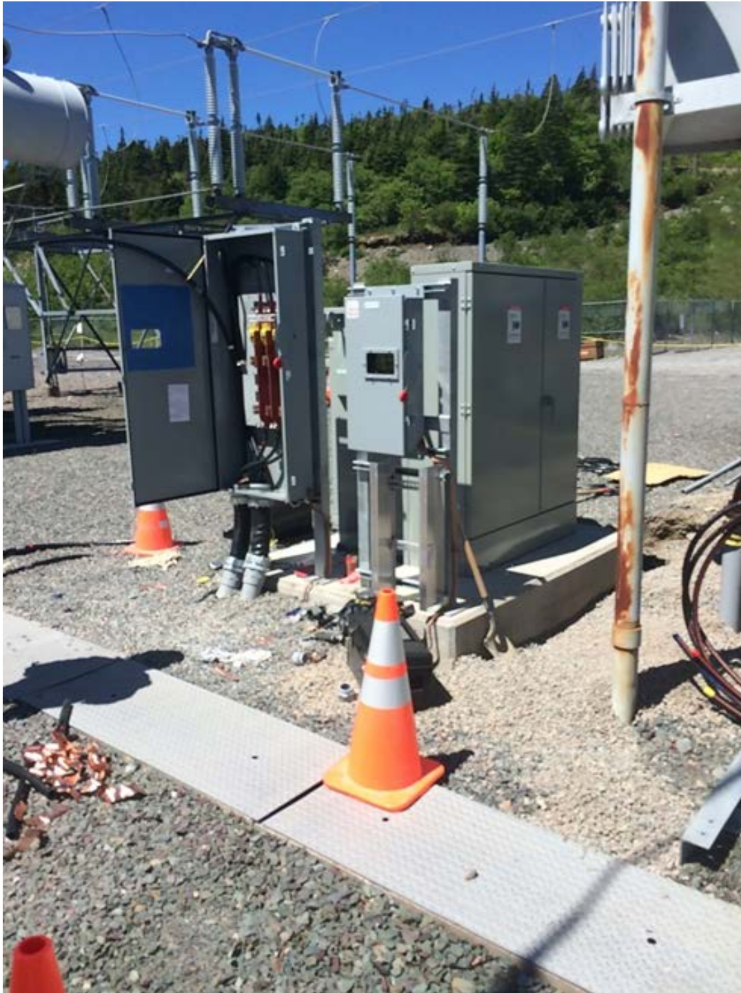
Western Avalon Terminal Station – Station Service Transformer on Pad
