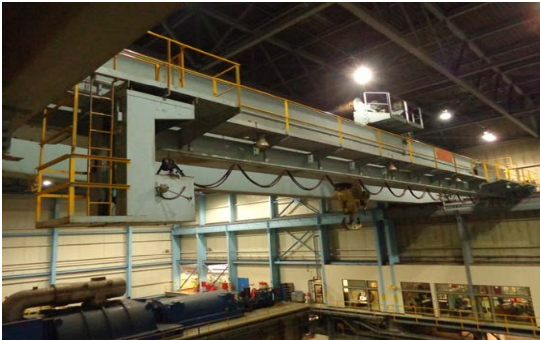
Figure 1: Overhead Crane 1 in Holyrood Powerhouse Turbine Hall
