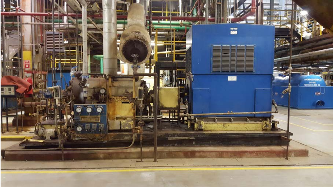
Figure 1: Unit 2 Boiler Feed Pump
