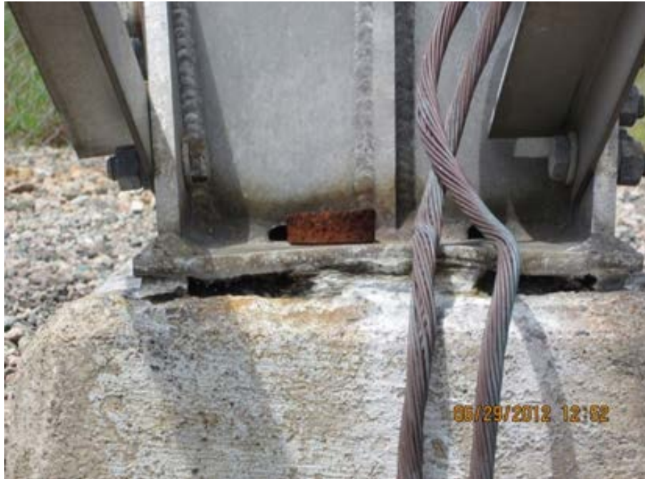
Figure 2: Example of Deformation of Baseplate Due to Aluminum Oxide Uplift
