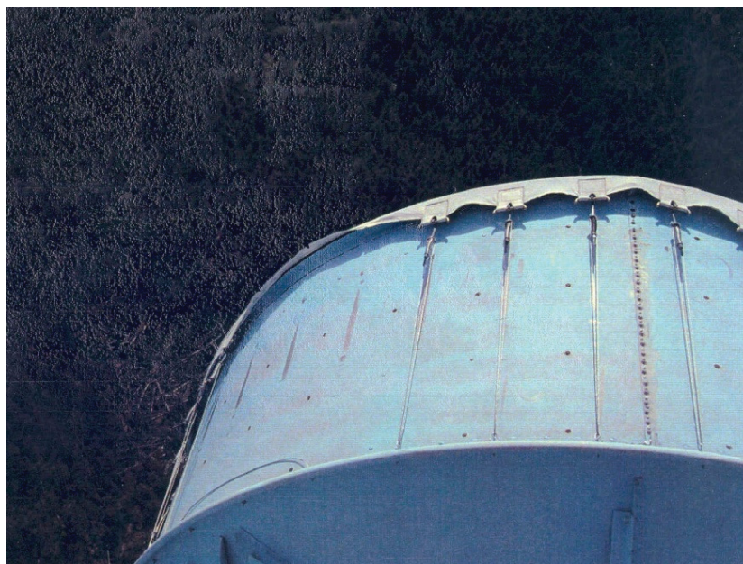
Figure 4: Missing Radome Mounts
